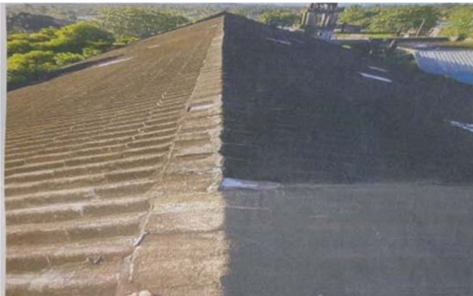
This is the OLD CHURCH ROOF
